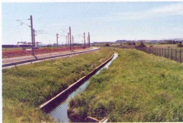
Photo 1 Vue du canal avant travaux View of the channel before the works
