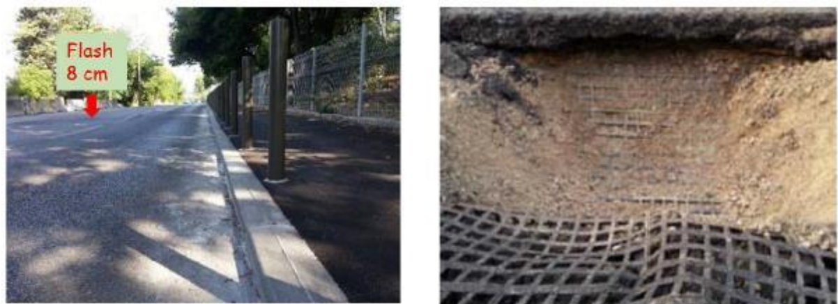
Figure 21 : Subsidence obtained in 2015 over an area reinforced using geosynthetic - Source: Trois Luc in La Valentine, Delmas and Gourc, 2017
