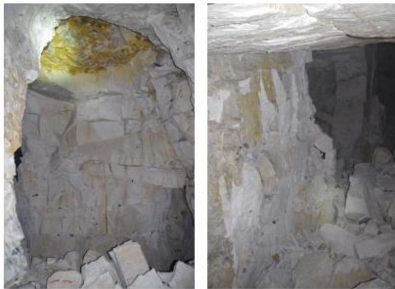
Figure 4 : Deteriorations in an underground quarry - Source: Ineris
